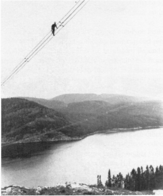
Figure 25.7a Four bundled conductors make up this phase of a 3-phase, 735 kV line. (Courtesy of Hydro-Québec)
